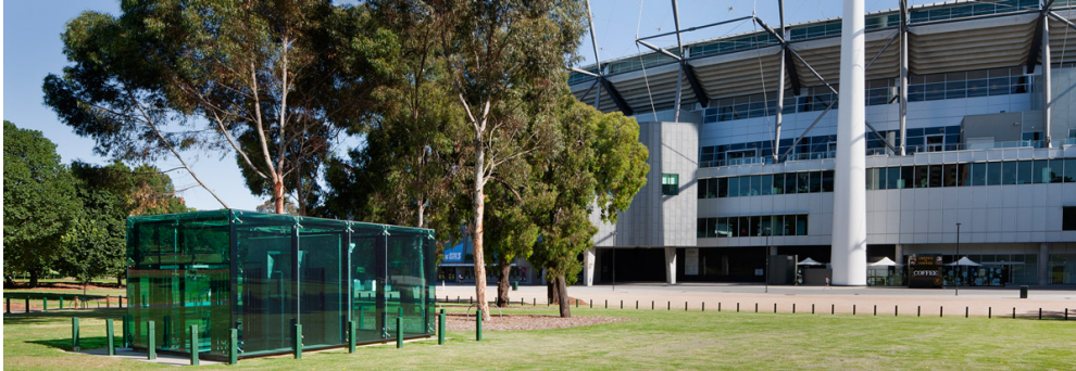
Treatment Plant within the MCG grounds. The plant is located underground but treated air is expelled to the open space. The surrounding open space is irrigated with recycled water.
