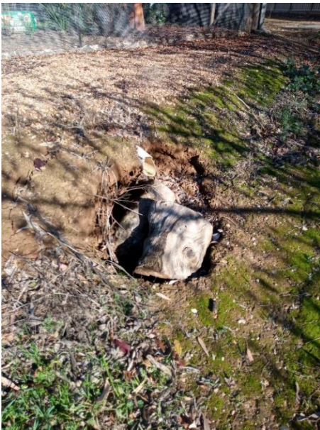
Photo – Private landholder pipe installation causing erosion
